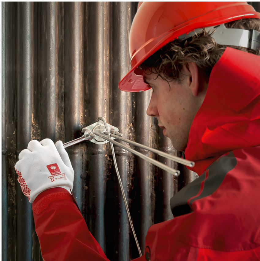
Figure 4.1.1 Industrial heat flux sensor mounted on a boiler wall using tack-welded threads and spring-loaded bolts. The sensor is mounted on a well prepared flat surface. Cabling must be provided with strain relief.
