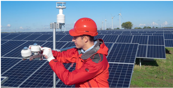
Figure 1 Two SR30 Class A pyranometers measuring GHI (Global Horizontal Irradiance) and POA (Plane of Array) in a PV performance monitoring system. How many systems should there be on such a power plant?
