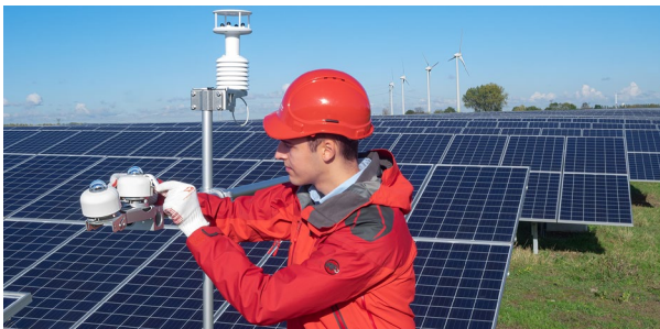
Figure 2 Two SR30 Class A pyranometers measuring GHI (Global Horizontal Irradiance) and POA (Plane of Array) in a PV performance monitoring system.
