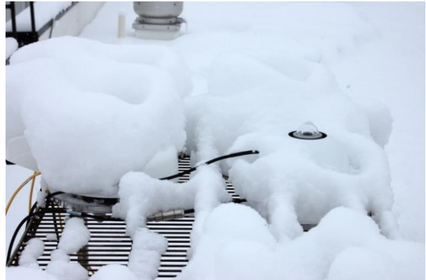
Figure 5 Does external ventilation work to remove snow? Not reliably: this photo shows 3 ventilation units in FEB 2014 in Logan UT, USA powder snow. Only 1 of the 3 pyranometers, the one at the right (SR20 with VU01), is visible. The other 2 are still covered in snow. Photo courtesy of Apogee Instruments Inc.
